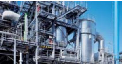
▲ Diphyl® flash system with a total output of 20 MW at 360^{\circ}\text{C} supplying process heat to a DMT plant in Germany.
